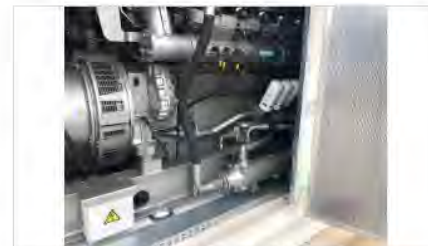
CHP Propane Engine
